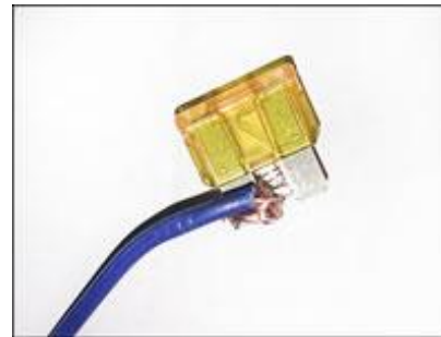
Wire Jammed Into a Fuse
