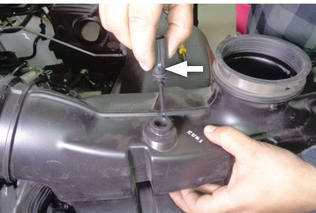
9. Remove IAT sensor from resonator, remove o-ring from IAT sensor then retain sensor for re-use.
